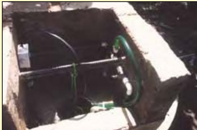
The completed "pump house." The electrical connections are on the left, the plumbing is on the right, and the pump is hanging from the bar in the middle.
