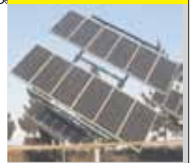
UTRF168 photo Installation by Miller Power and Communications Atascadero, CA
